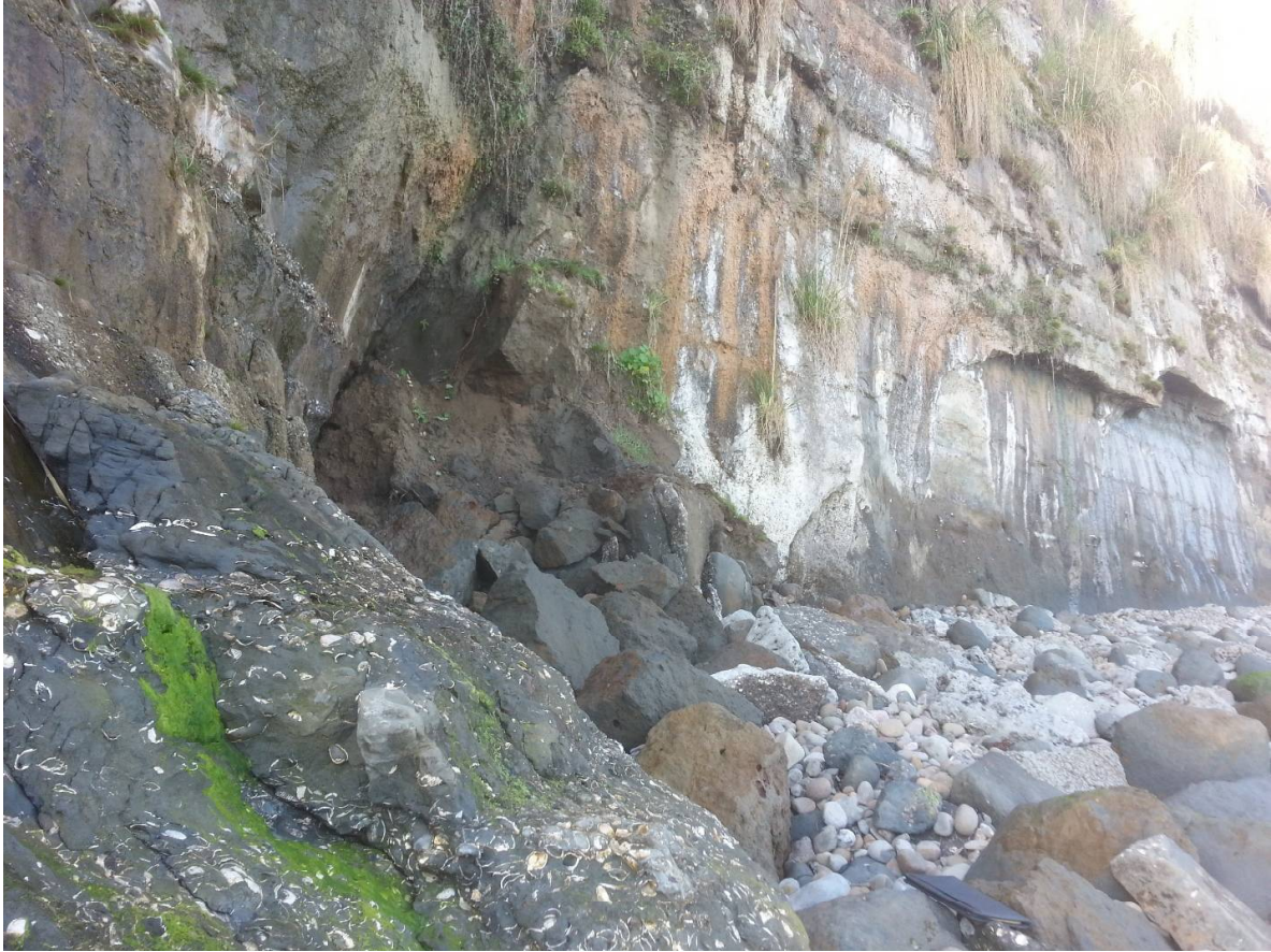
Close Up View of Rockfall Also Shows Bedrock Outcrop at Base of Bluff Just Upcoast
