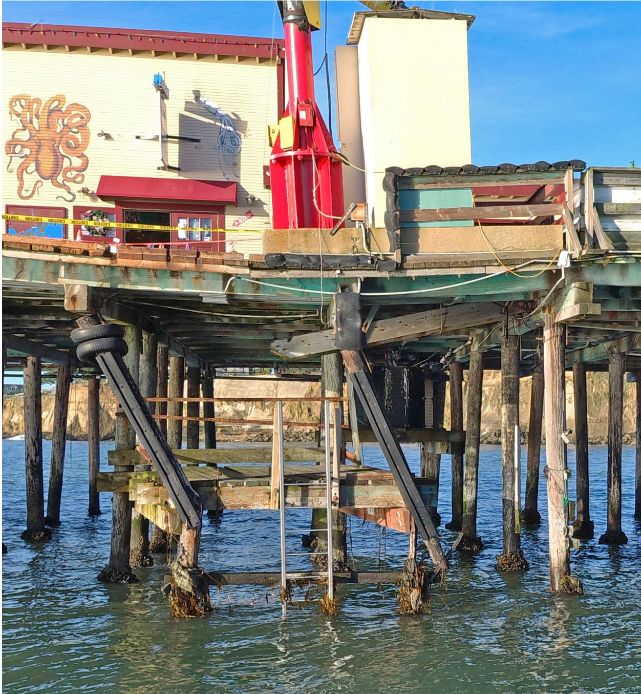
Broken pilings below the boat hoist are causing the wharf to sag.
