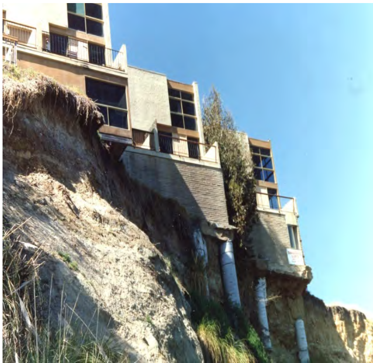
Figure 12a - Cliff Erosion Beneath Apartments on Depot Hill (c. 1984)
