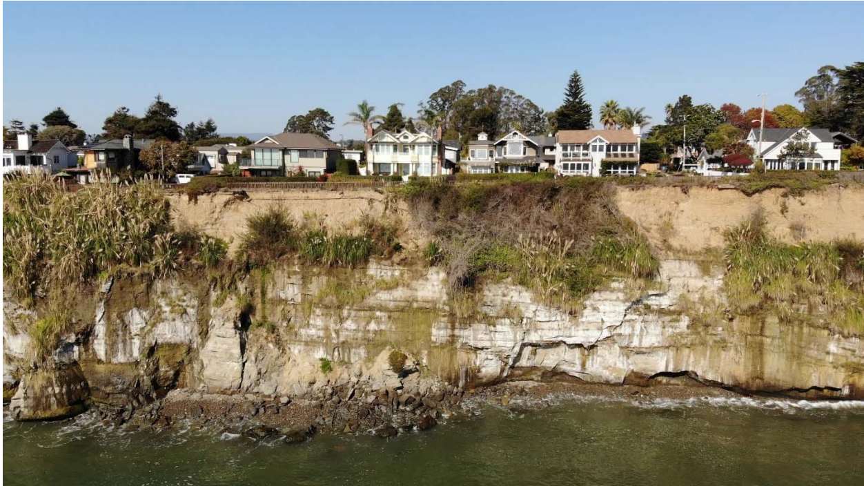
April 17, 2017 drone photo of Grand Avenue pathway at time of closure due to risk of further slope failure
