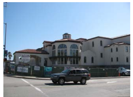
There are two hotels in the Plan area: the Best Western (top) and the Fairfield Inn & Suites (bottom), which opened in July 2011.
