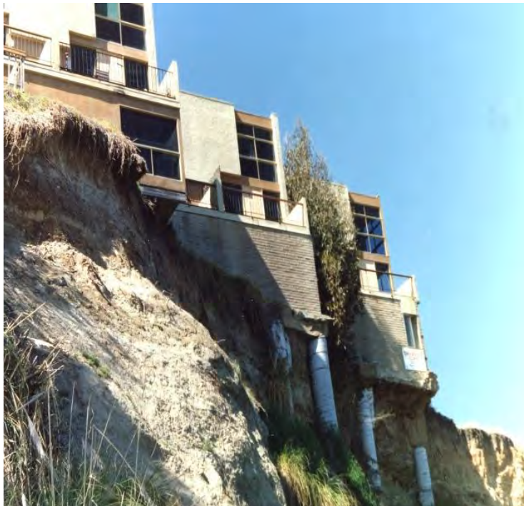
Figure 12 - Cliff Erosion Beneath Apartments on Depot Hill (ca. 1964)
