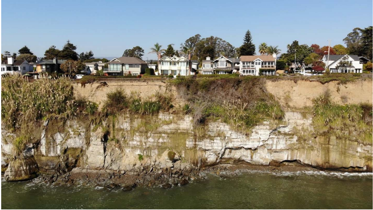
April 17, 2017 drone photo of Grand Avenue pathway at time of closure due to risk of further slope failure
