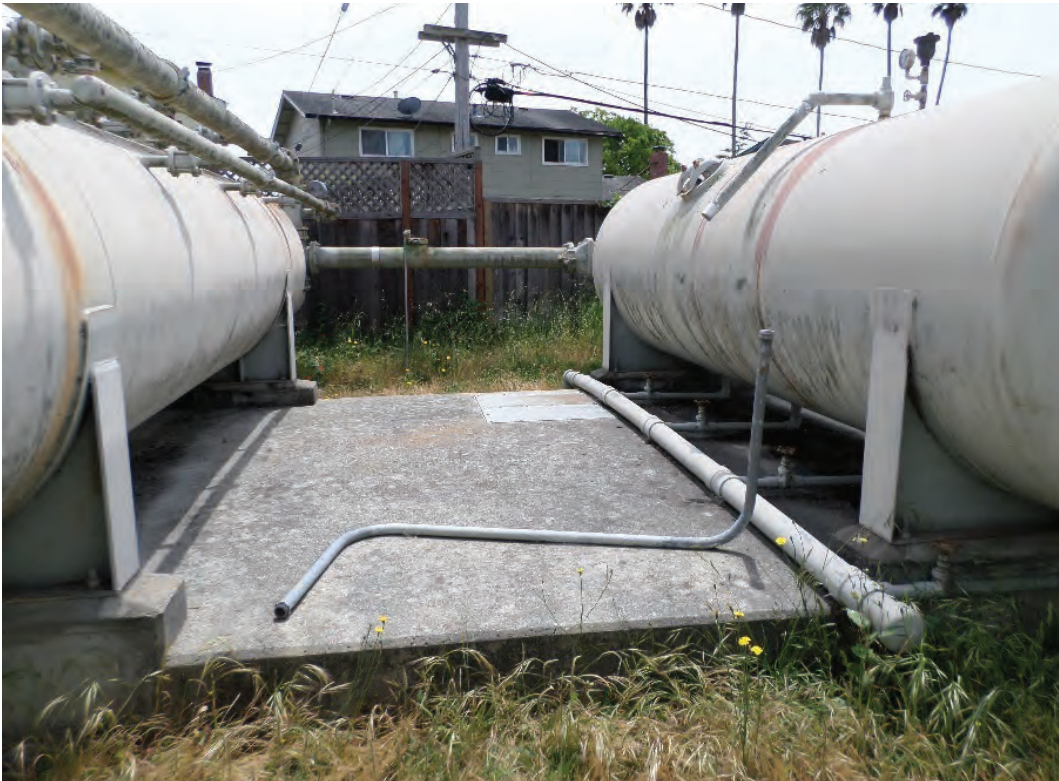
Figure 5 - Monterey Avenue Well Site - Existing water treatment vessels and underground concrete basin, as viewed from within existing perimeter fencing.
