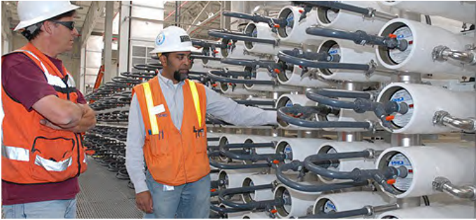
Orange County Water District's Groundwater Replenishment System has produced over 200 billion gallons of purified water and has been in operation for 40 years. (photo credit: Orange County Water District)
