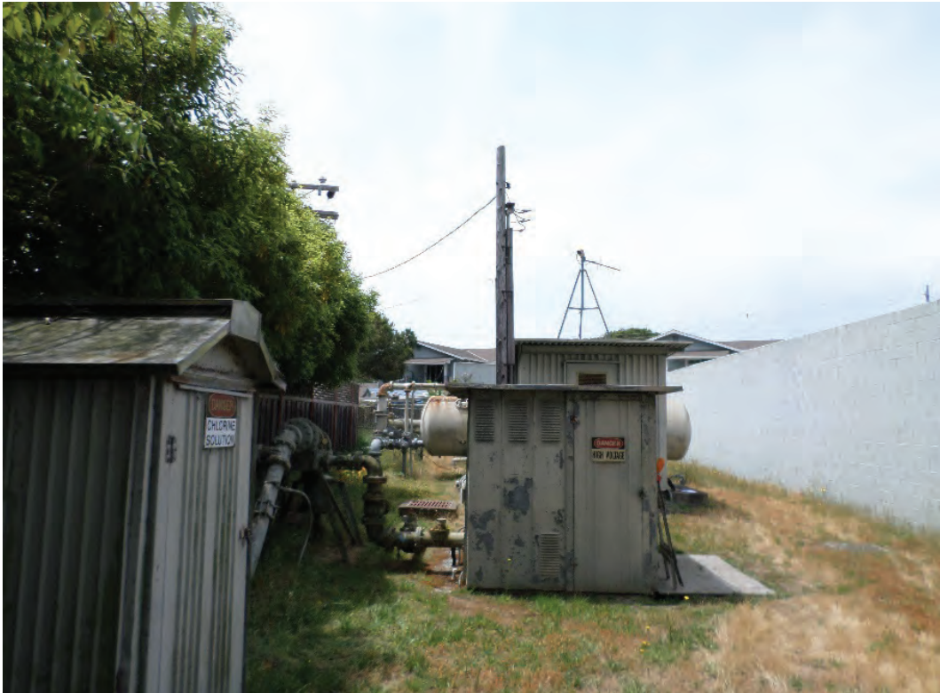
Figure 4 - Monterey Avenue Well Site - Existing chlorine, electrical control, and well enclosures and power pole, as viewed from within existing perimeter fencing.
