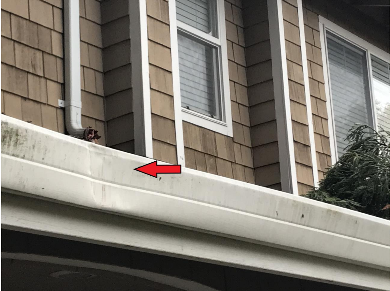
Where the branch hit roof.
