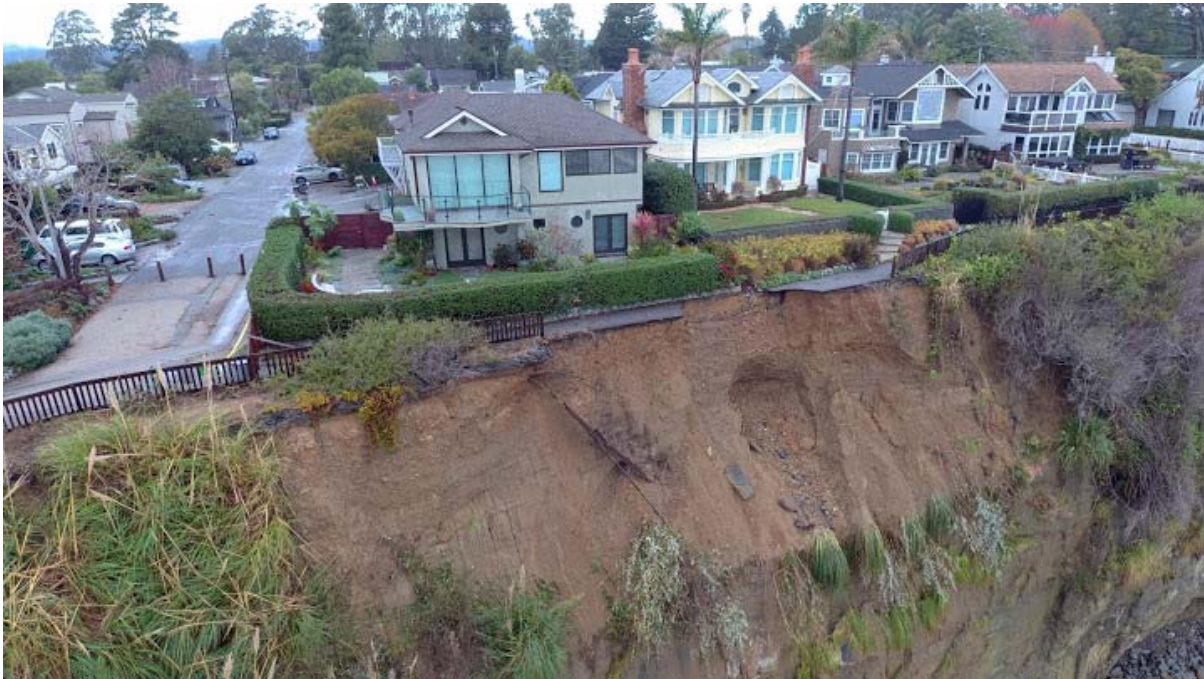
December 4, 2019 drone photo of slope failure along Grand Avenue pathway. Oakland Avenue to the left of photo.
