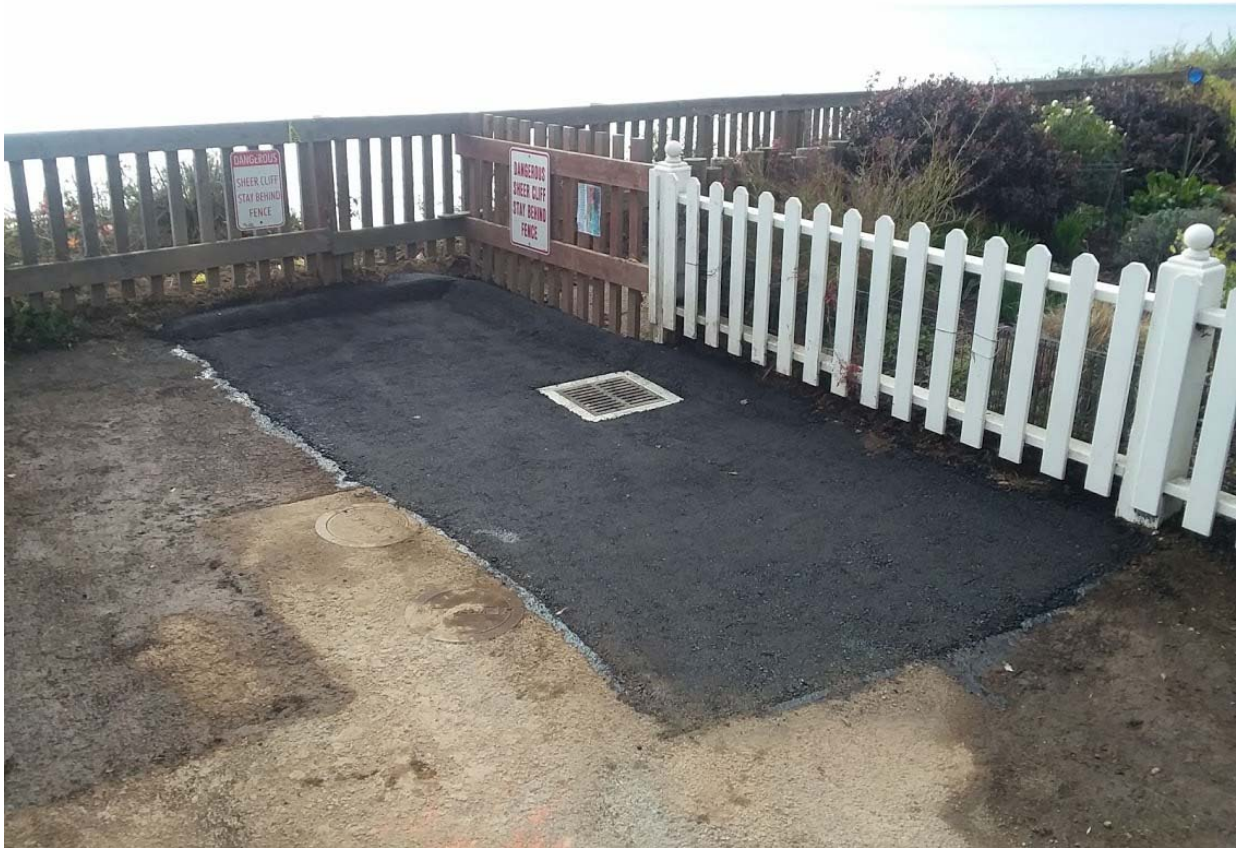
New drainage inlet at the end of Hollister Avenue constructed under emergency declaration
