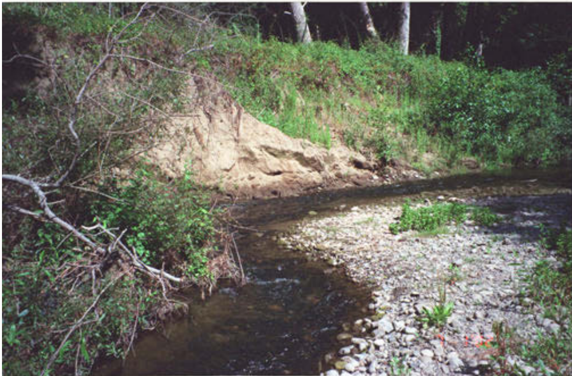
Photo 20. Eroding Streambank on Soquel Creek in the Nob Hill Reach Above the Lagoon in 2002
