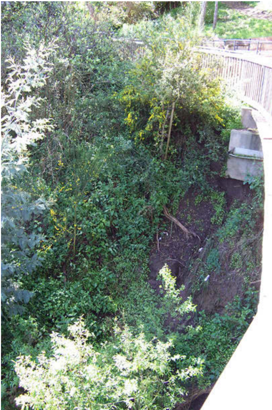
Photo 18. Undermined Peery Park Bridge Abutment
