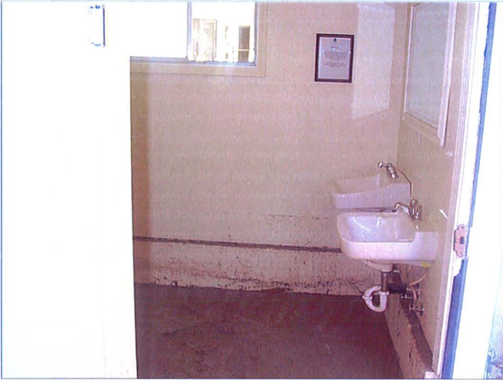
Flood damaged public restroom
