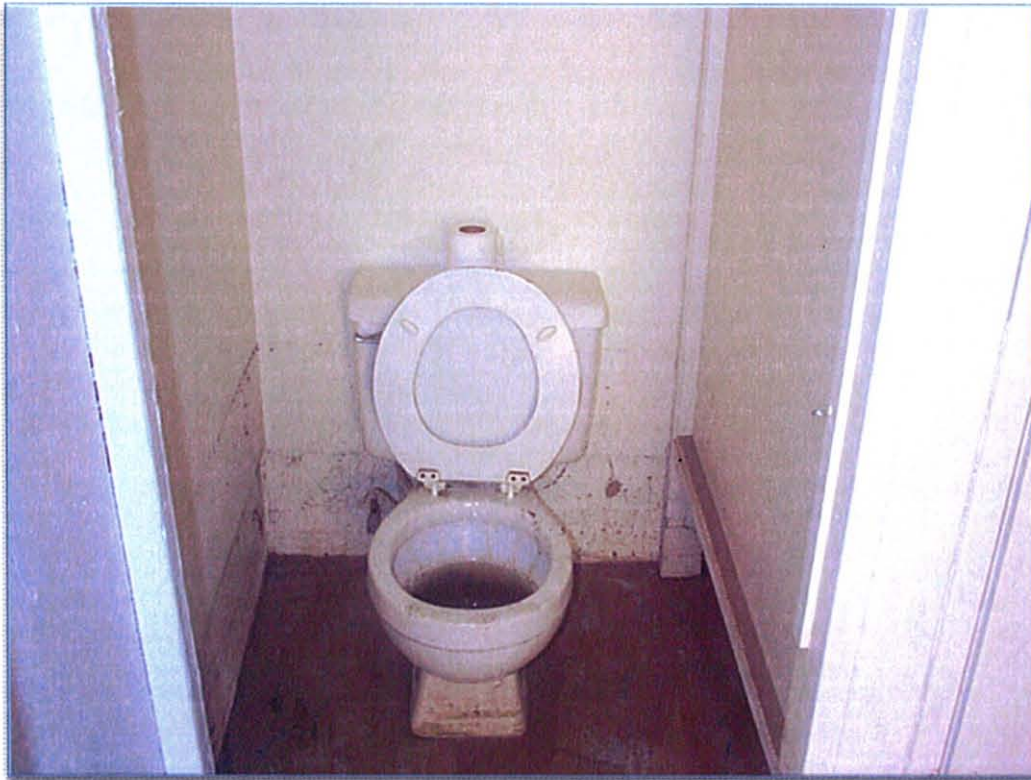
Flood damaged public restroom
