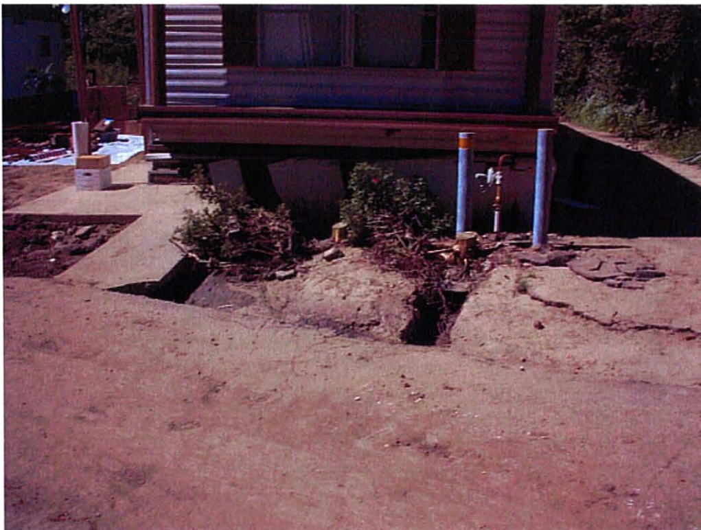
Soil washed away under and around home destroying landscape and walkway
