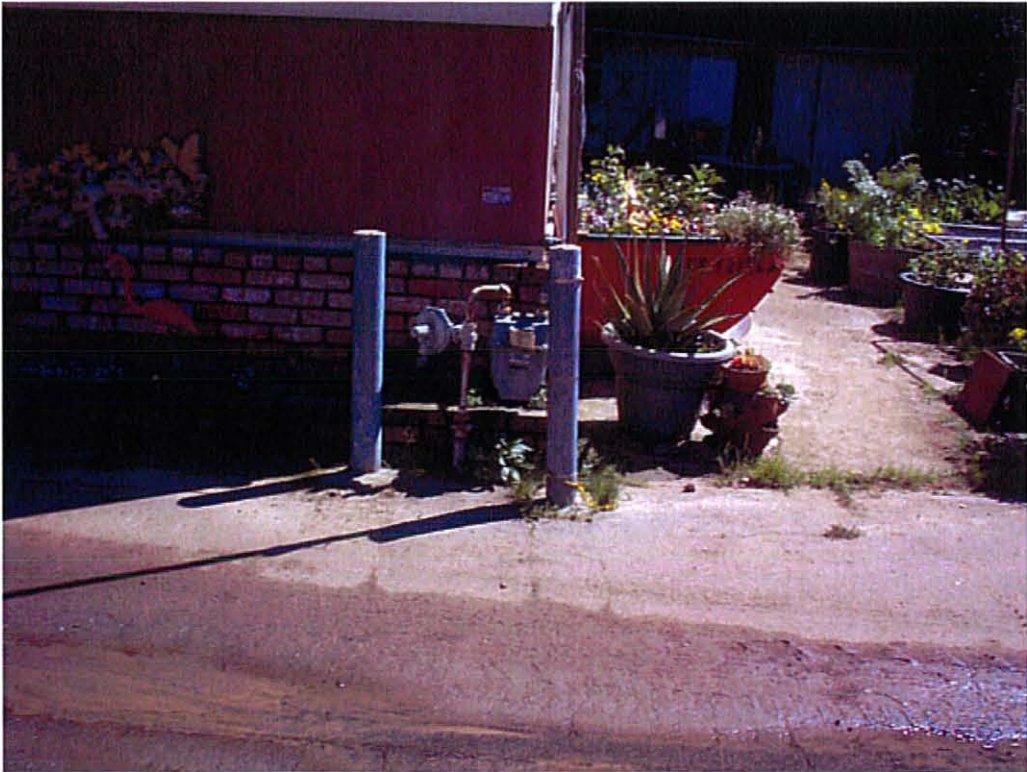
Typical gas meter installation
