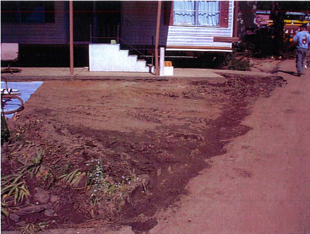
Damaged car parking spaces adjacent to mobile home
