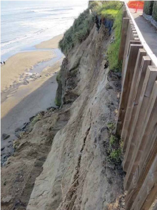
Recent Failure between Oakland and Hollister Avenues (directly upcoast from Sacramento Avenue)
