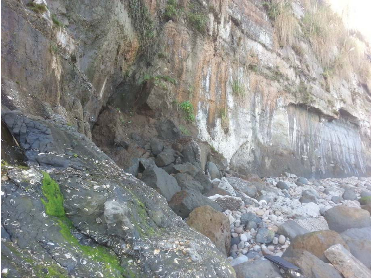
Close Up View of Rockfall Also Shows Bedrock Outcrop at Base of Bluff Just Upcoast
