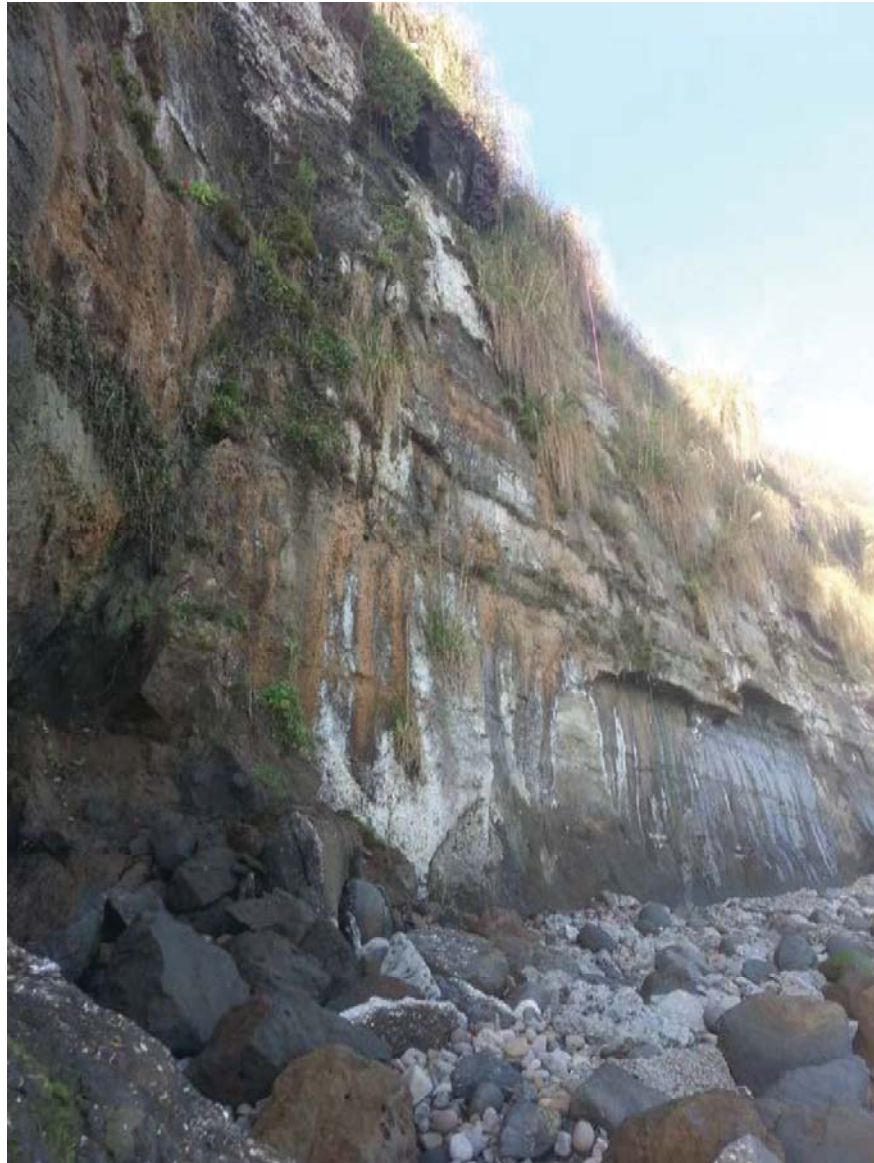
Bluff Face Looking Downcoast Showing Rockfall at Left (Not on Property)
