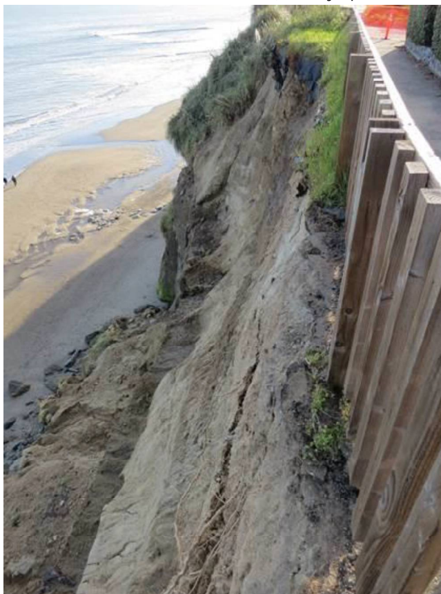
Recent Failure between Oakland and Hollister Avenues (directly upcoast from Sacramento Avenue)
