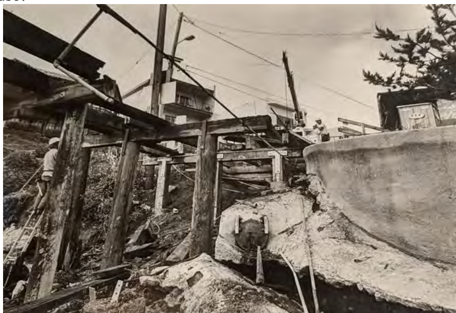
Green Sheet Photograph of the 1981-82 Repairs at Wharf Road, facing north. Courtesy Capitola Historical Museum
