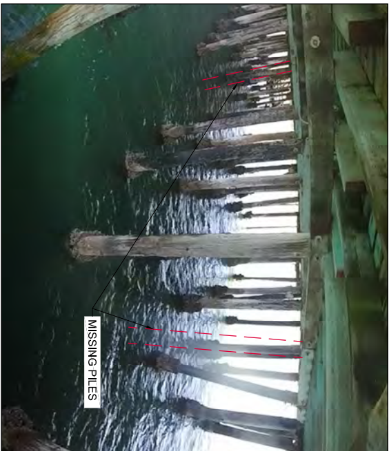
PHOTO 7 MISSING TIMBER PILES BELOW RESTAURANT
