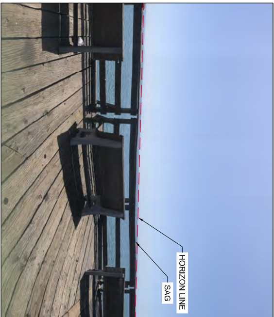
PHOTO 8 SAG IN WHARF STRUCTURE
