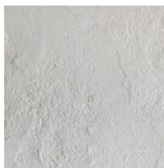
3 (E) EXTERIOR STUCCO TO REMAIN, (N) WHITE OR LIGHT-GRY PAIN COLOM, T.B.D.
