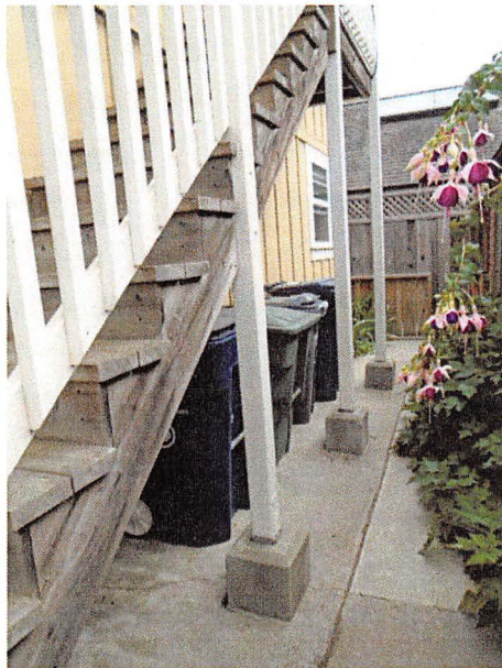
Trash storage under staircase
