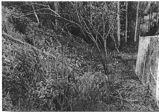
Fill Slope Bordering the SCWD Parcel (right) and the McGregor Park Parcel (left)
