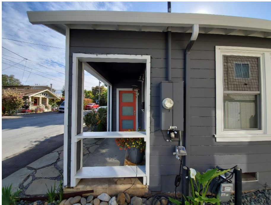
Detail of Front Porch and West Elevation. Viewed facing east. Showing concrete porch floor, exposed rafter tails, v-groove siding and altered door and windows. May 2020. (Photo by Matthew Orbach, City of Capitola)
