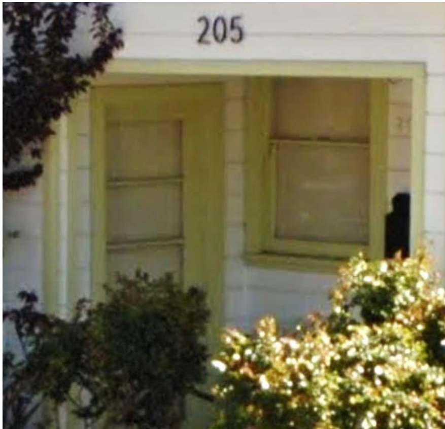
Detail of Front Porch Corner. Viewed facing southeast. Illustrating horizontal lites on west-facing door and dog ears on upper window sash prior to renovations. (Google Streetview, accessed May 2020)
