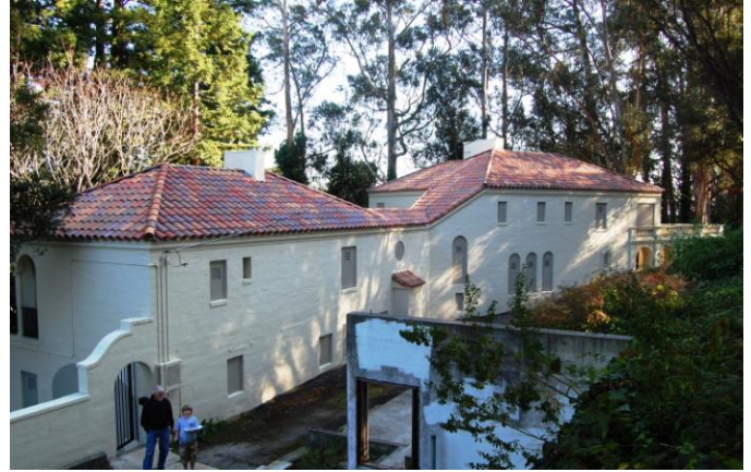
Capitola Public Works employee Ed Morrison showed off the work done so far on the Rispin preservation project to museum trustee Niels Kisling in December 2011.
