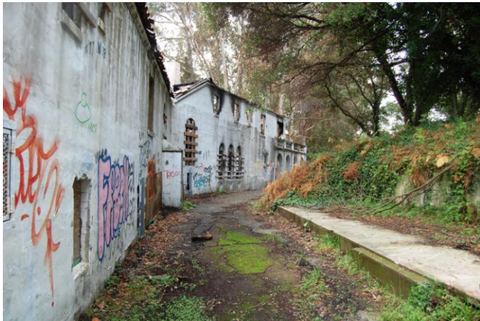
In this photo taken in January 2010 the graffiti is evident. Harder to see, but just as disheartening, is the missing roof that was burned in the vandalism fire of May 2009.
