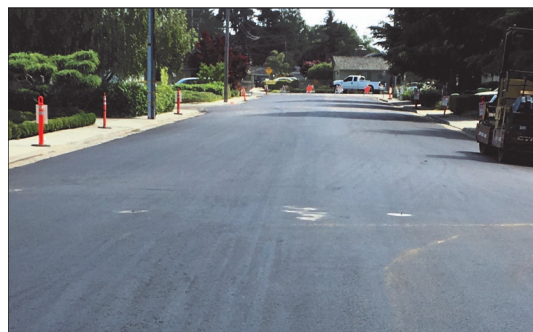
From top: Ozzi’s Memorial Dog Park at McGregor, Stockton & Esplanade improvements, Rosedale paving
