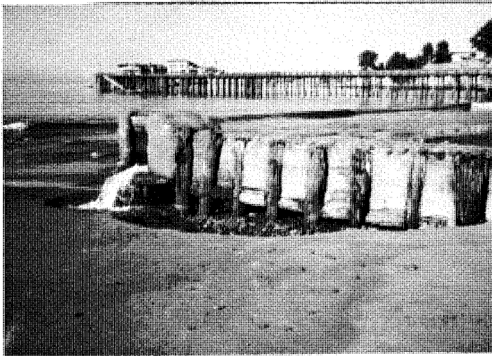
Seepage Under Flume Plugged with Sand Bags 14Jul95
