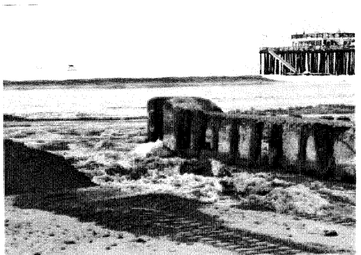
Flume Draining as Channel Cuts Through Sandbar 14Jun95
