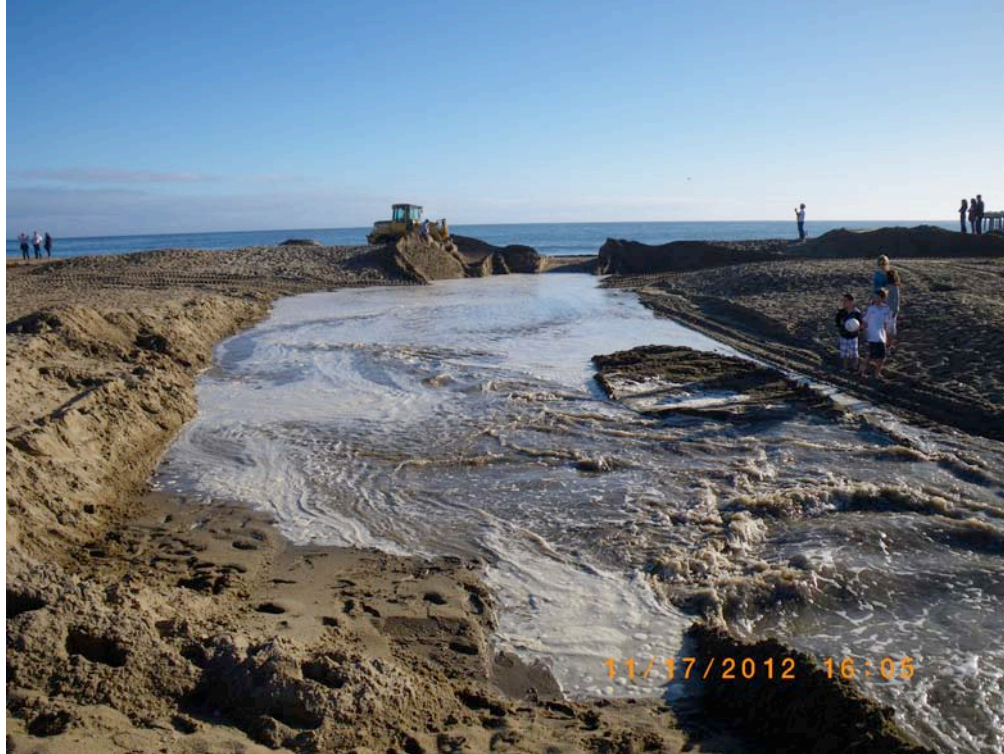
Facilitated sandbar breaching procedure (inner berm breached and outer berm reinforced). 17 November 2012.
