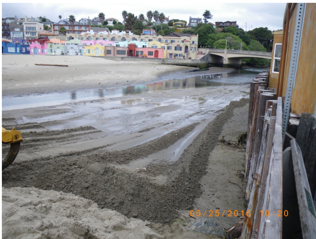
Lagoon deepened adjacent to restaurants (work done above estuary water surface) 25 May 2016
