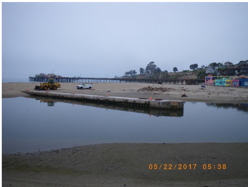
Exposed flume prior to sandbar construction. (Add 1 hour to time stamp.) 22 May 2017
