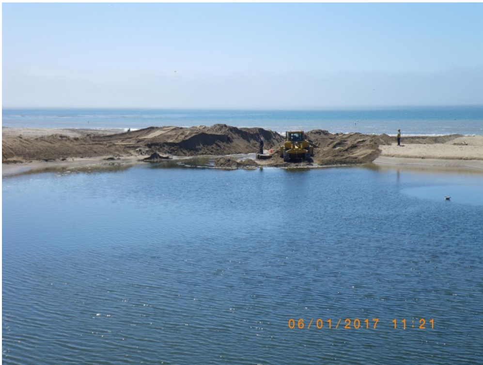
Work to firm up sand and prevent seepage began around flume inlet. 1 June 2017
