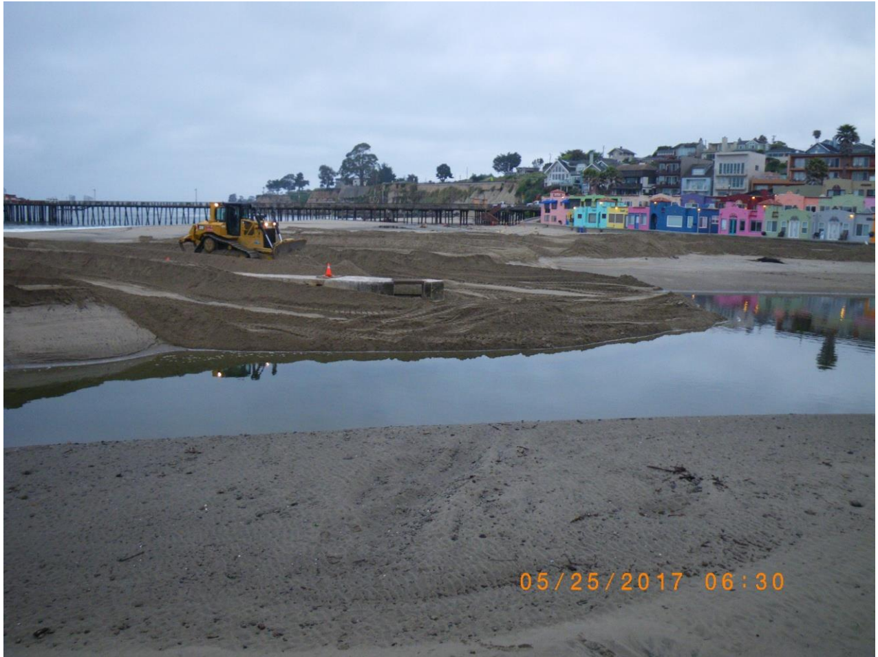
Compacted pad of sand constructed around flume inlet. Outlet channel in foreground. 25 May 2017
