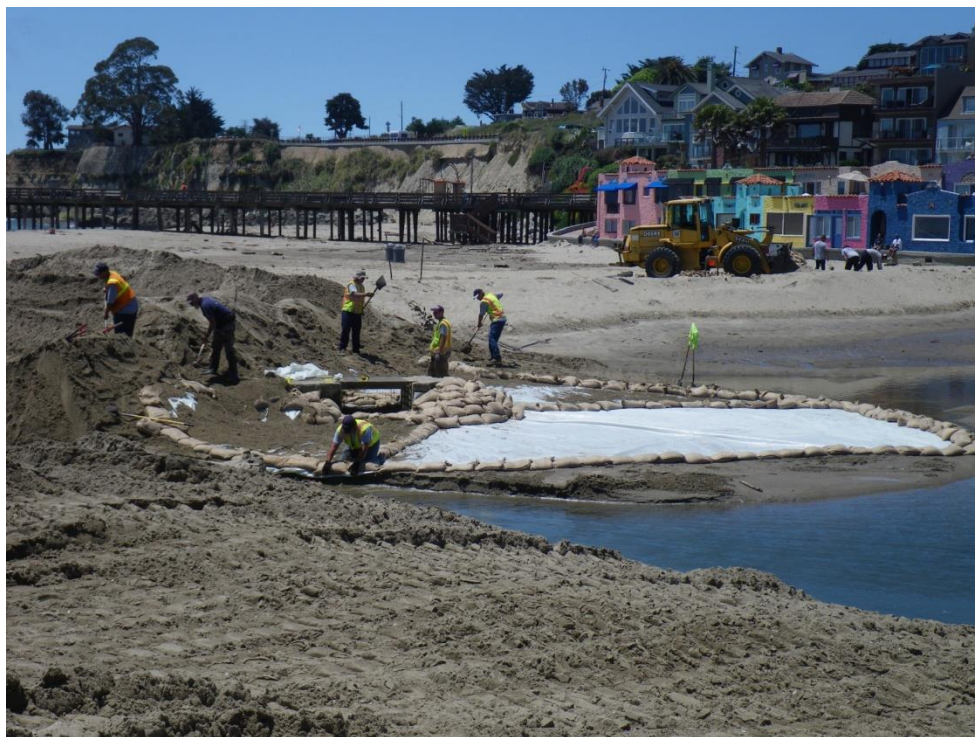
Preparation of pad around flume inlet to prevent seepage. Outlet channel in foreground. 1 June 2017
