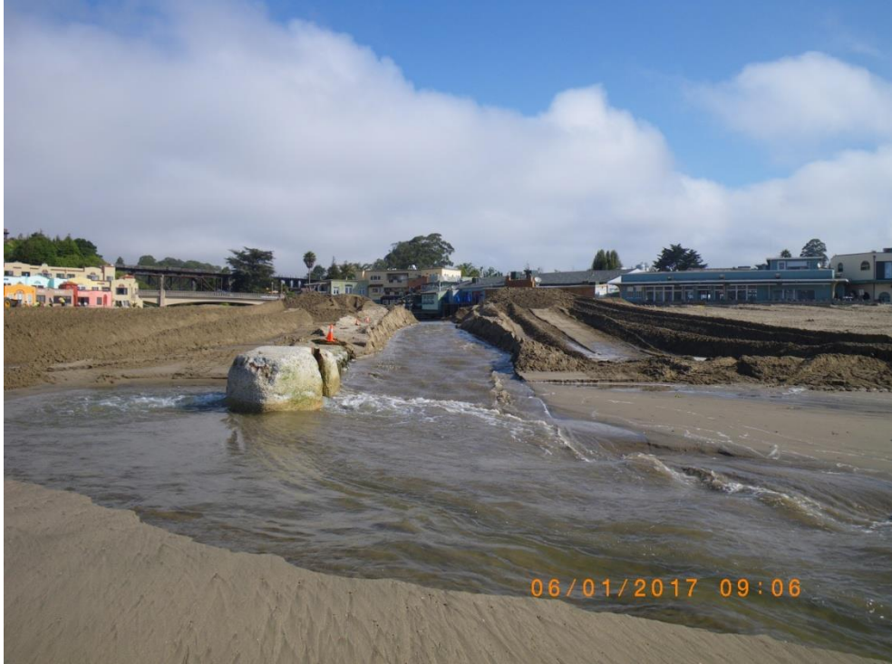
Outlet channel along east side of flume after manual breaching of sandbar. 1 June 2017
