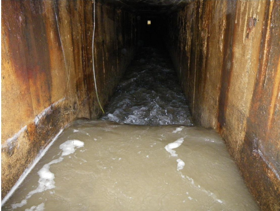
Weir intact inside the flume to maintain water depth at flume inlet. (Date stamp lost when flash was activated.) 1 June 2017
