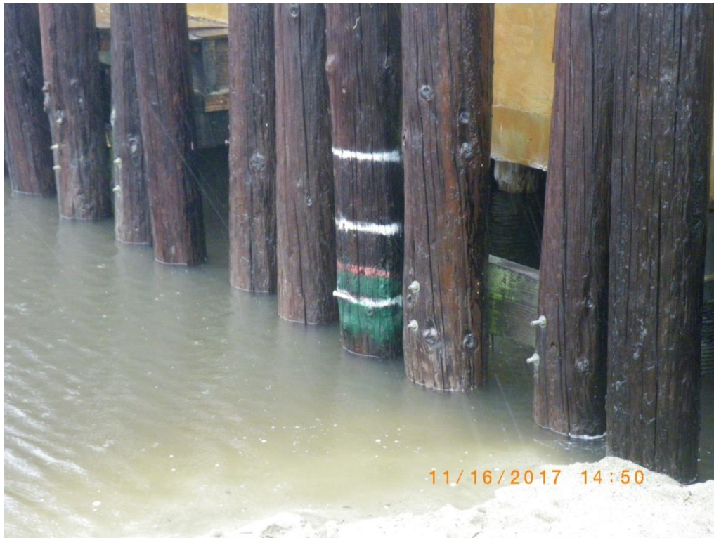
Lagoon Water Surface in Relation to lower piling ring with bent bolt, 40 minutes after facilitated emergency breach. (Subtract 1 hour from time stamp.)
