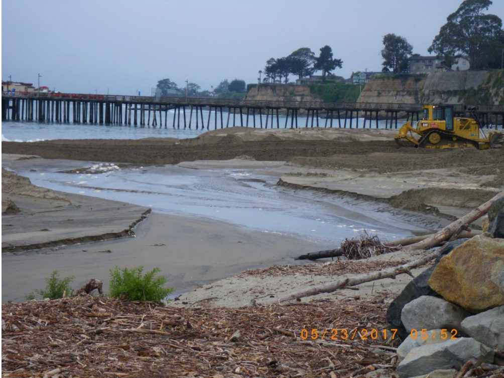
Streamflow from flume exit had meandered over to lateral channel overnight. Pathway was re-directed to Bay. (Add 1 hour to time stamp.) 23 May 2017
