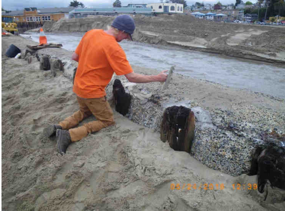
Public Works Maintenance Worker, Cooper Sanden, filling cracks in the flume. 24 May 2018
