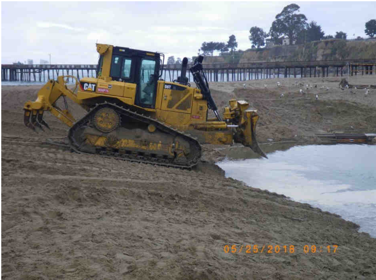
Public Works Heavy Equipment Operator, Matt Kotila, compacts lagoon margin with bull-dozer. 25 May 2018
