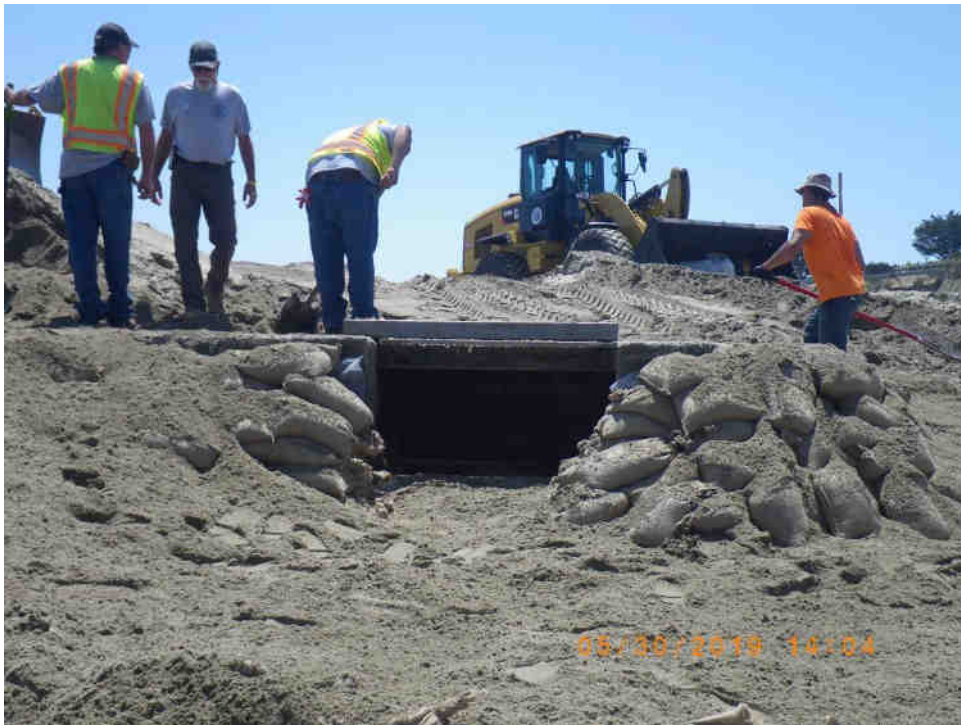
Sandbags placed around the flume inlet to prevent leakage of sand along the flume after sandbar closure. 30 May 2019
