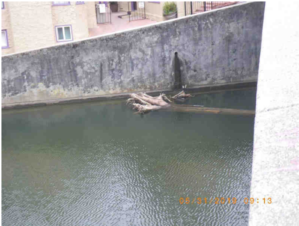
Log secured near Stockton Avenue Bridge. 31 May 2019
