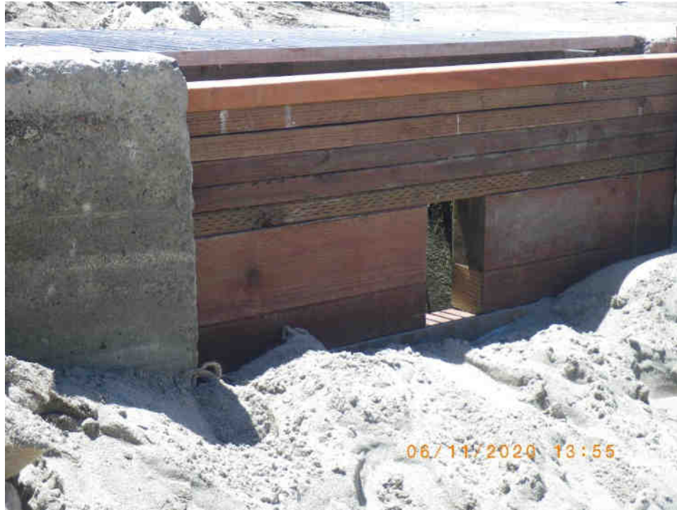
Underwater portal constructed with flashboards installed to the top of the flume inlet. 11 June 2020
