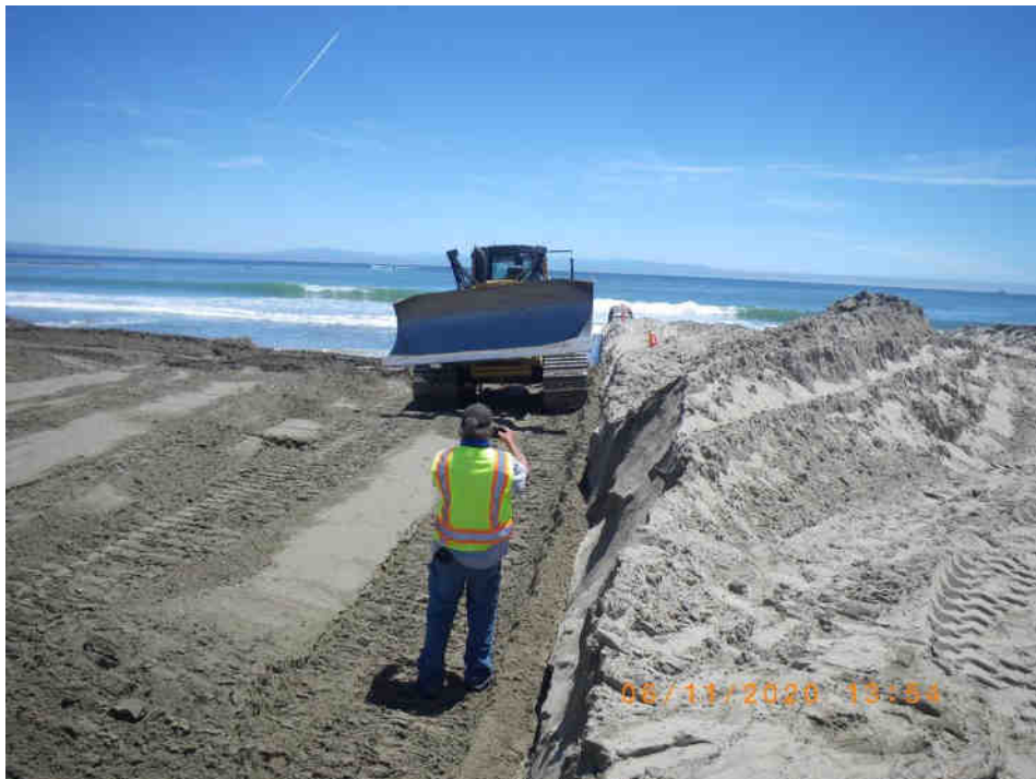
Kotila packing sand under and beside the flume during sandbar closure to reduce seepage from the lagoon to the Bay. 11 June 2020
