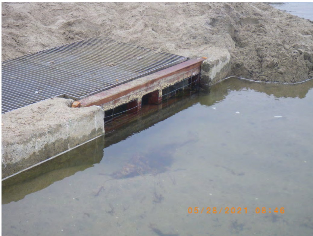
Water flowing over screened flashboards and through unscreened passage portal to provide steelhead passage to the Monterey Bay. 28 May 2021
