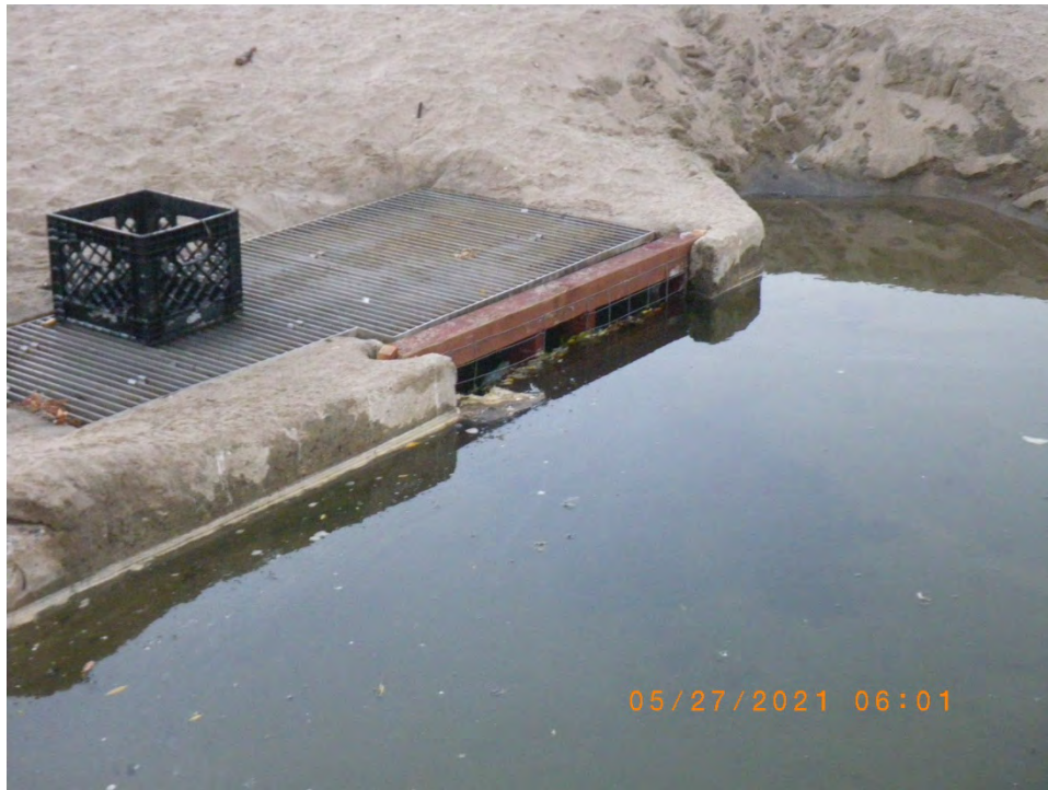
Lagoon filled overnight with added flashboards and screened frame having an unscreened steelhead passage portal in the center. 27 May 2021
