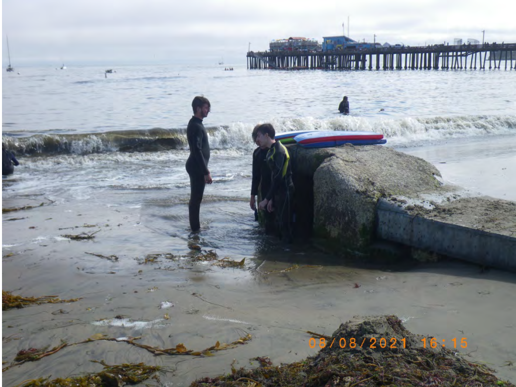
Flume outlet to the Capitola Beach and Monterey Bay. 8 August 2021
