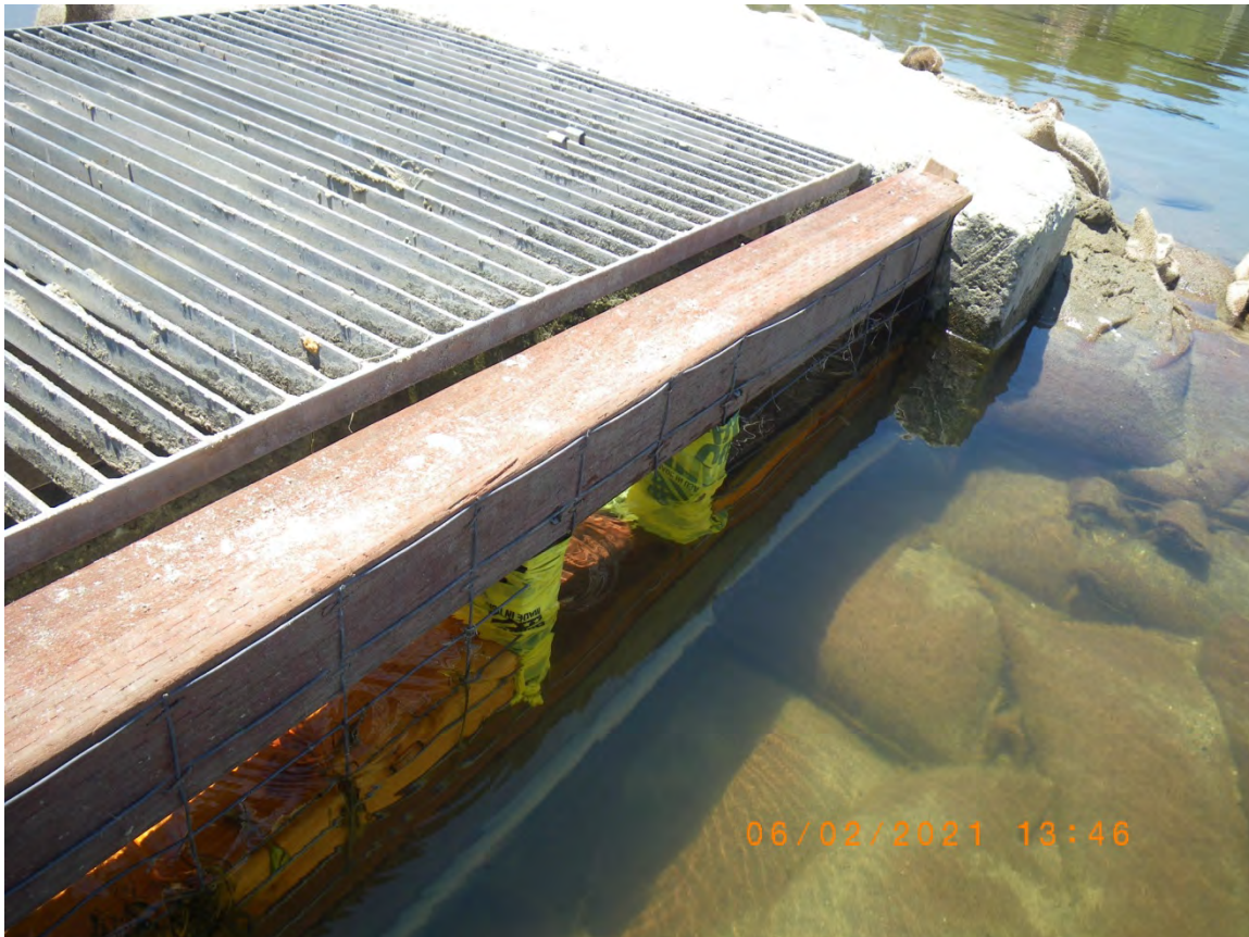
Water flowing over screened opening and through unscreened passage portal to provide adult and smolt steelhead passage to the Monterey Bay. 2 June 2021
