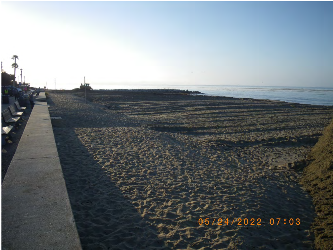
Lateral channel conversion to beach completed the previous day. Kotila filling in area near the jetty with sand that was lost by tidal action overnight. 24 May 2022
