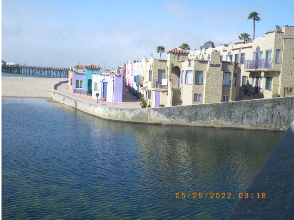
Venetian Court wall with deep water adjacent to it, immediately downstream of the Stockton Avenue Bridge. 25 May 2022
