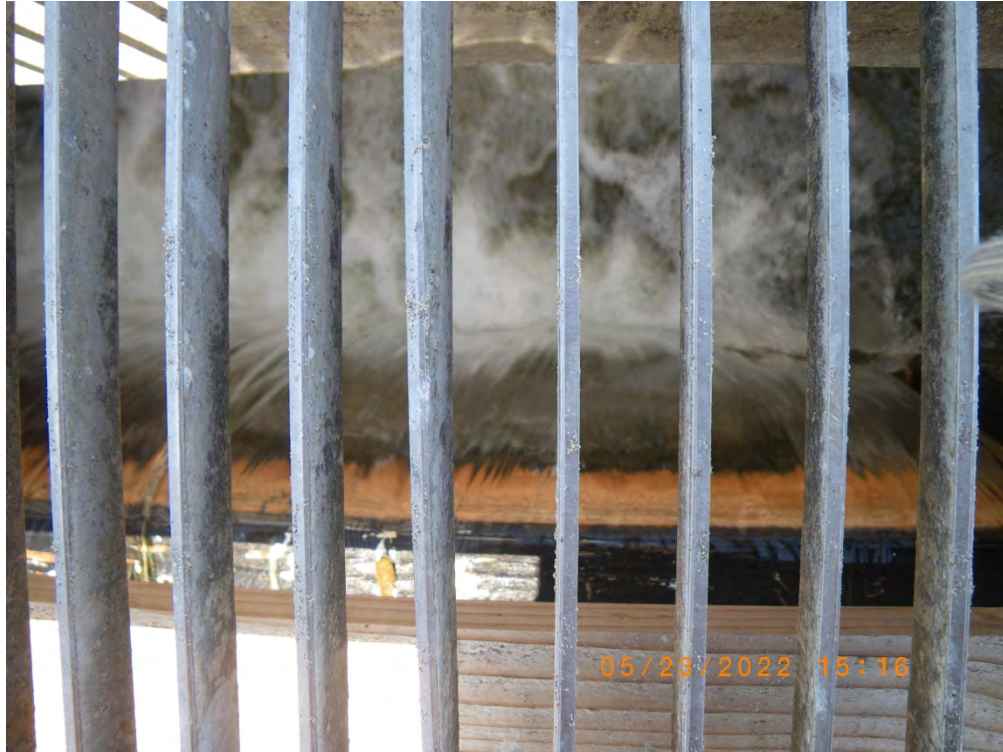
Water spilling over base of wooden frame into the flume inlet (looking from above) to provide steelhead access to Monterey Bay. 23 May 2022
