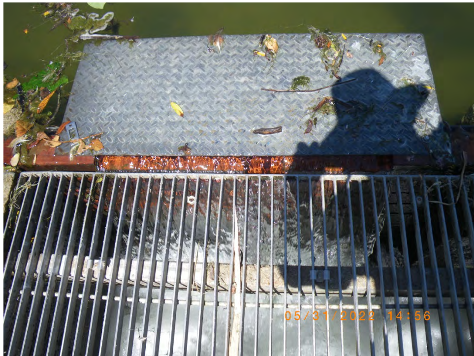
Lagoon spilling over top flashboard and smolt passage notch under shroud. 31 May 2022
