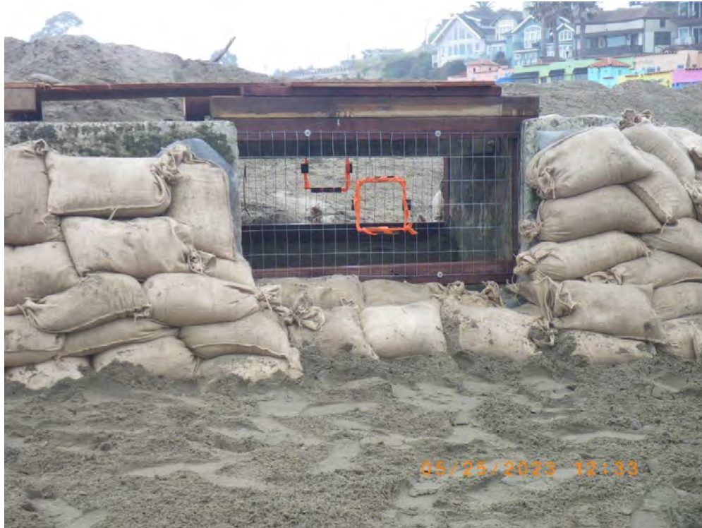
Screen installed in flume inlet with underwater portals. 25 May 2023
