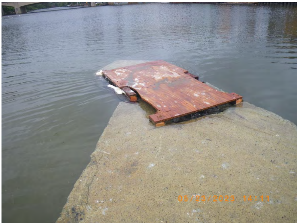
Screened flume inlet covered with plywood because steel plate and grate were lost over the winter. 23 May 2023 (Replacement steel grate installed by 24 June 2023)
