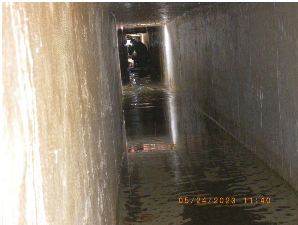
Cooper Sanden inspects the flume for cracks in the epoxy lining. 24 May 2023
