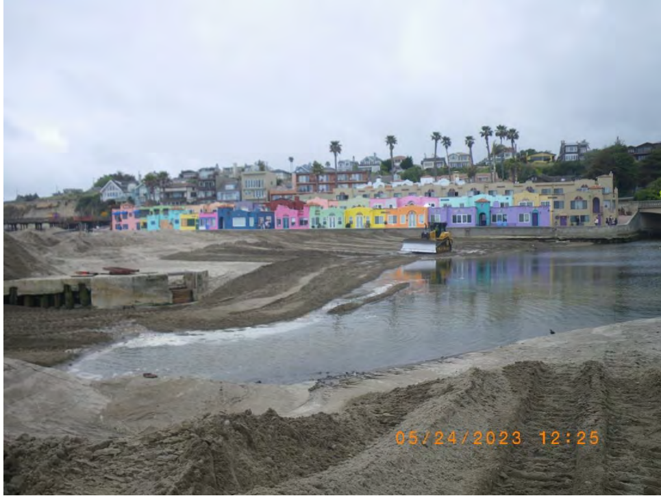
Kotila contouring western lagoon bottom and flume inlet pad above the water line during estuary drawdown. 24 May 2023
