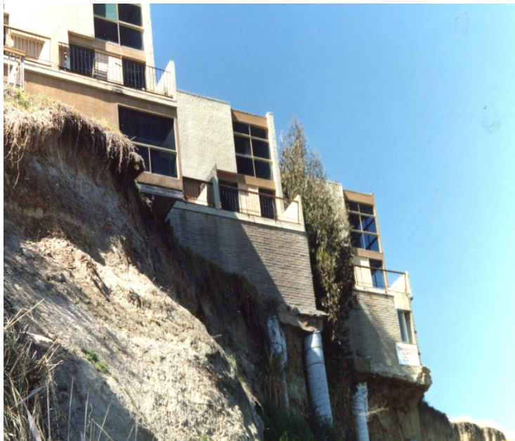
Figure 12 - Cliff Erosion Beneath Apartments on Depot Hill (c. 1984)
