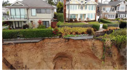
Figure 12b – Grand Avenue Pedestrian Pathway Erosion
