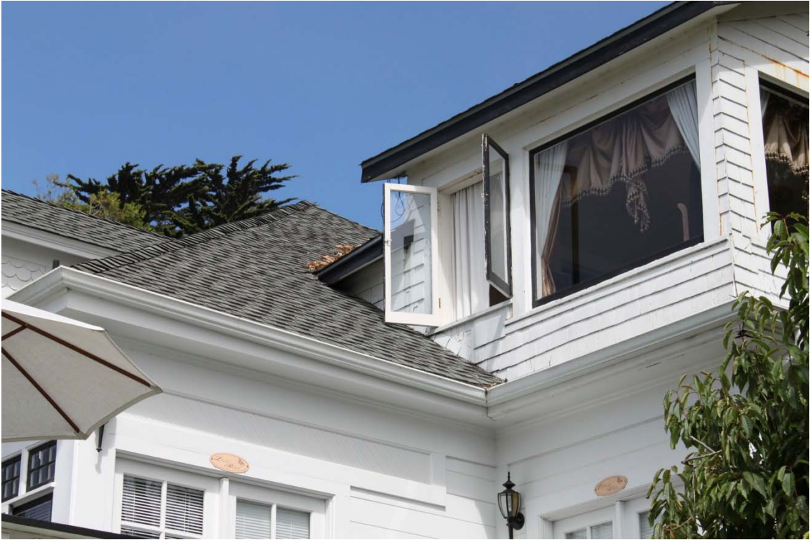
Main house, detail of second-story addition, view looking northwest (Architectural Resources Group, July 2013)
