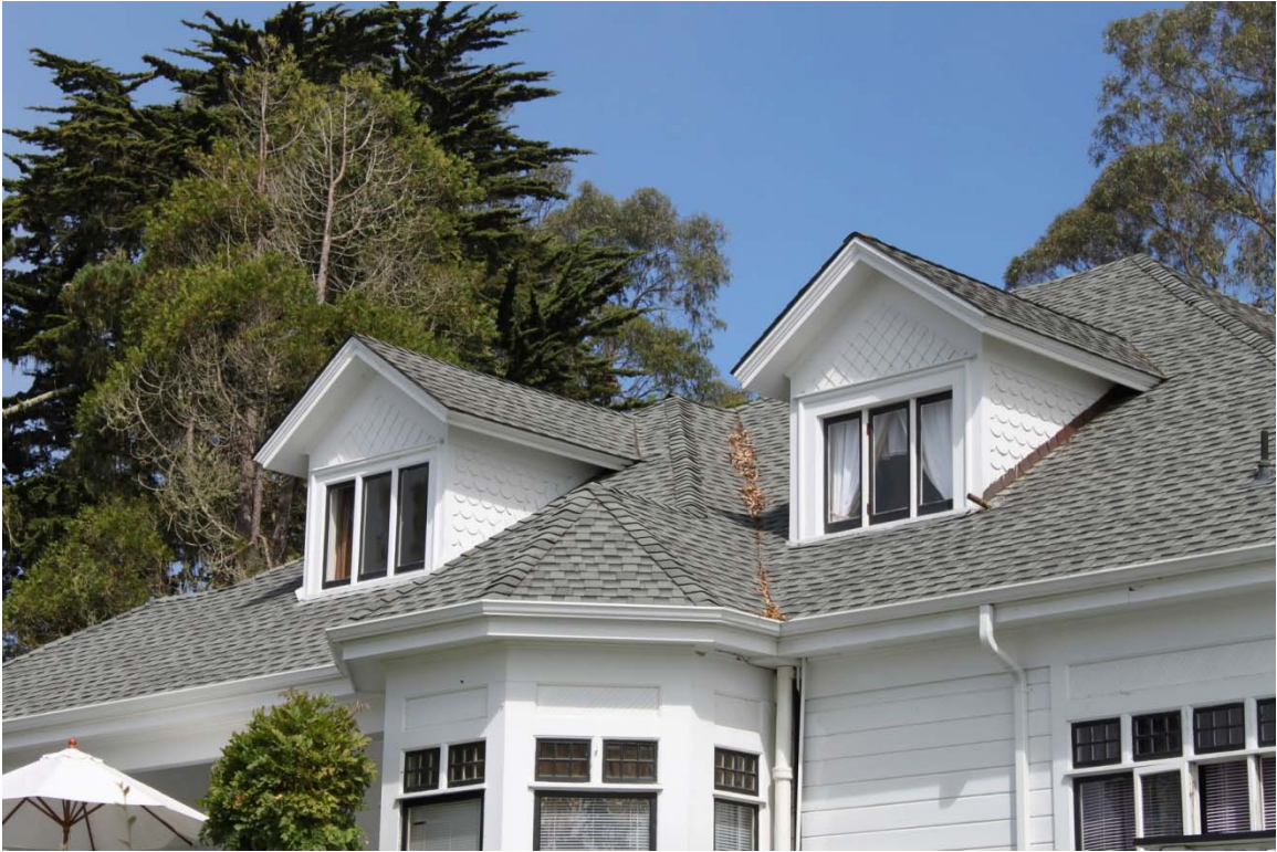
Main house, south elevation dormers, view looking northwest (Architectural Resources Group, July 2013)
