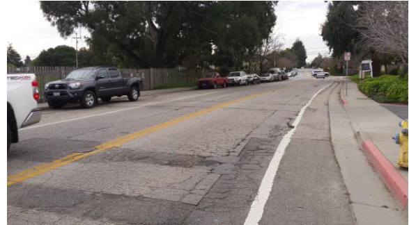
Area east of 38 th Avenue intersection showing potholes, patches, and alligator cracking.
