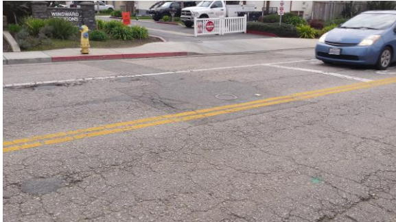
Area east of 38 th Avenue intersection showing severe alligator cracking and potholes.
