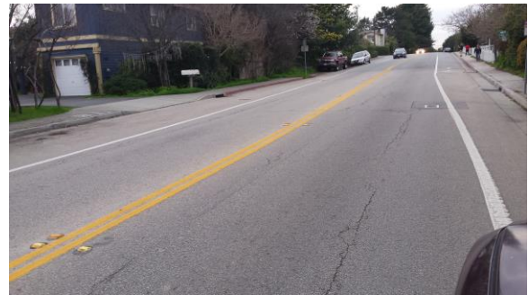
West of 38 th Avenue intersection showing some longitudinal cracking.
