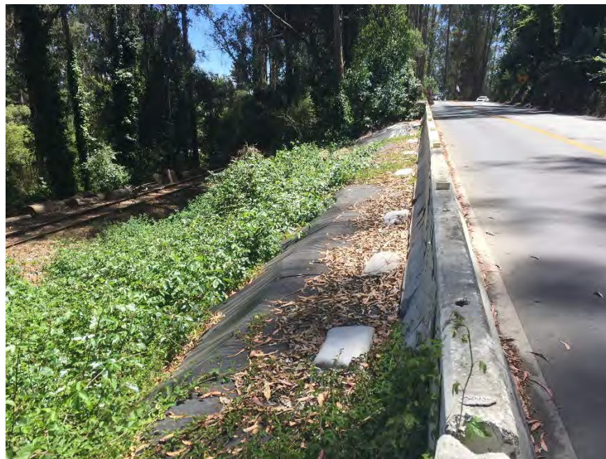
Photo 1. Slope Damage Along Park Avenue, taken July 7, 2018
