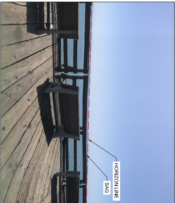
PHOTO 8 SAG IN WHARF STRUCTURE
