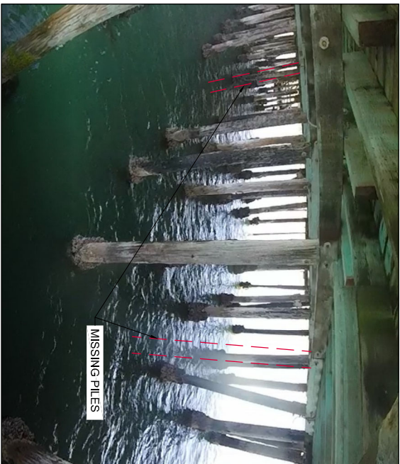
PHOTO 7 MISSING TIMBER PILES BELOW RESTAURANT
