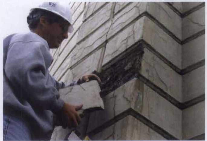
Figures 14. Layers of architectural concrete that have debonded (spalled) from the surface were removed from a historic water tank during the investigation performed to assess existing conditions. Photos: Anita Washko, Wiss, Janney, Elstner Associates, Inc.
