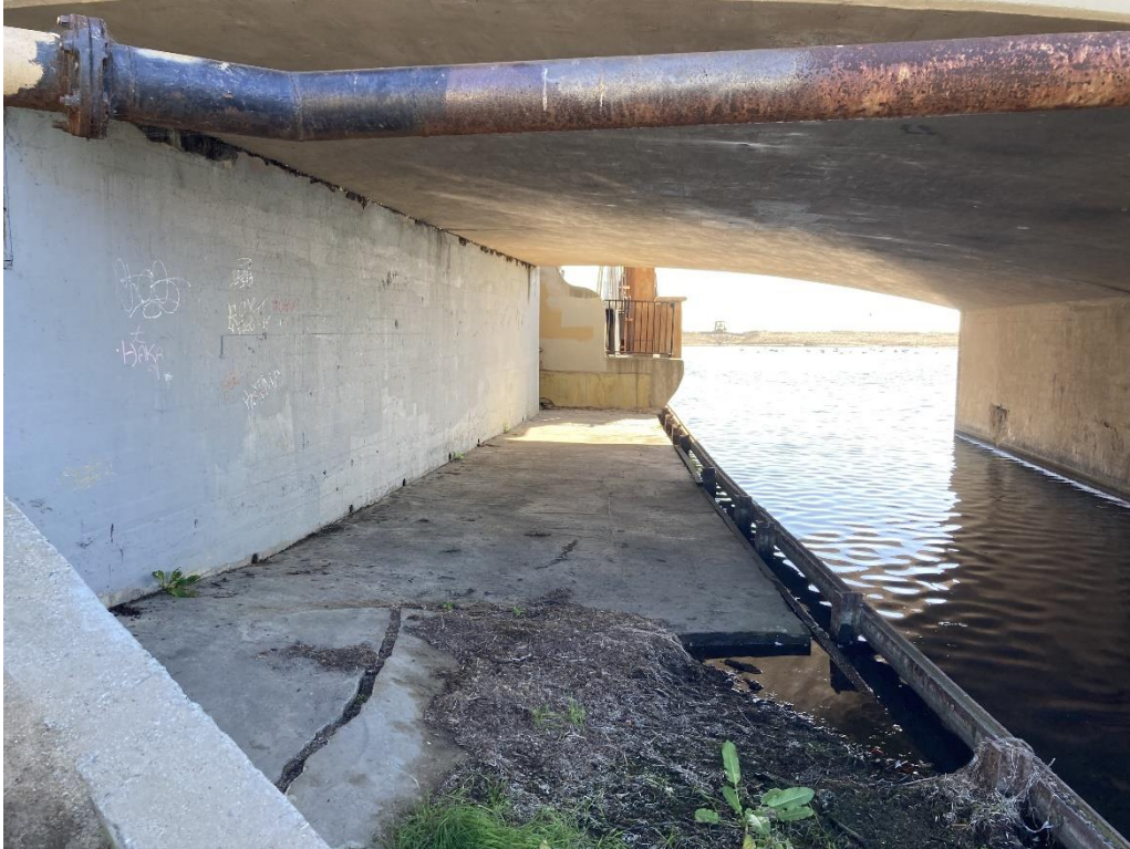
Figure 5. Detail of cracked concrete walkway on eastern side of Soquel Creek
