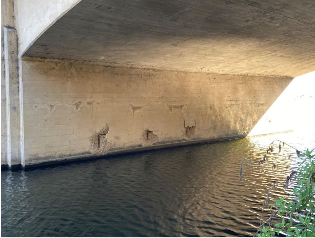
Figure 3. Detail of spalled concrete on West face section of West Pier
