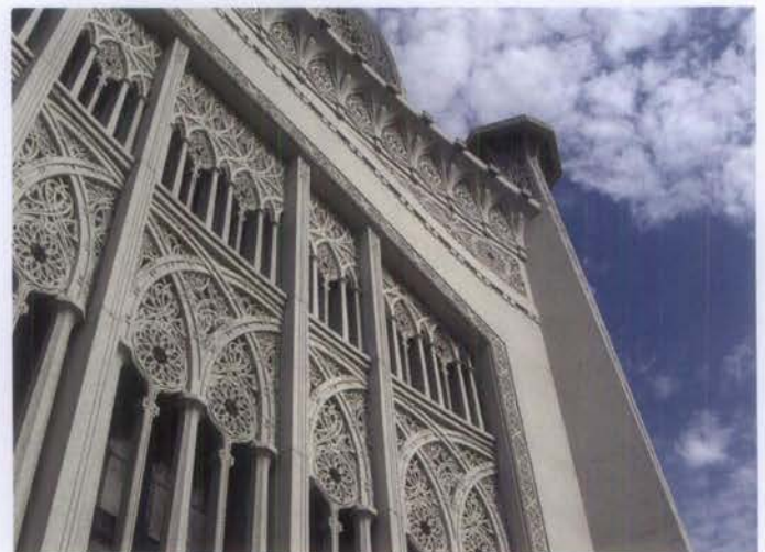
Figure 4. The highly ornamental concrete panels on the exterior facade of the Baha'i House of Worship in Wilmette, Illinois, illustrate the work of fabricator John J. Earley, known as "the man who made concrete beautiful."
