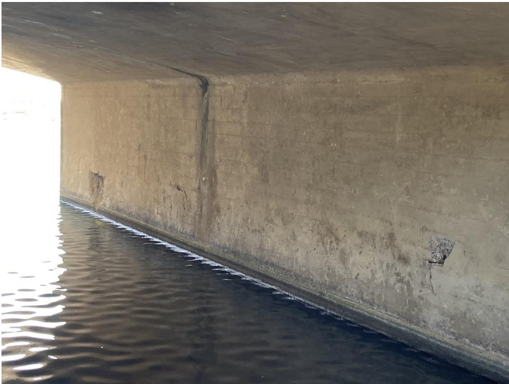
Figure 4. Detail of spalled concrete on East face section of East Pier
