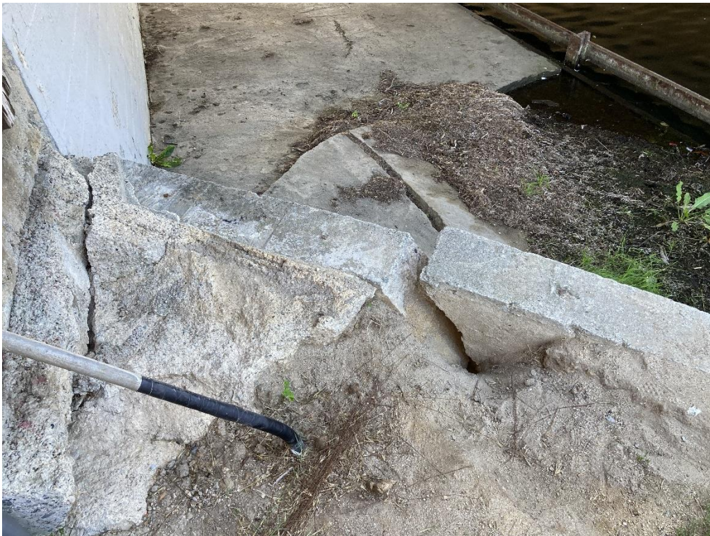
Figure 6. Detail of cracked concrete walkway and retaining wall on eastern side of Soquel Creek
