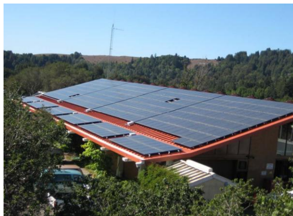
Solar panels on Graham Hill Water Treatment Facility
